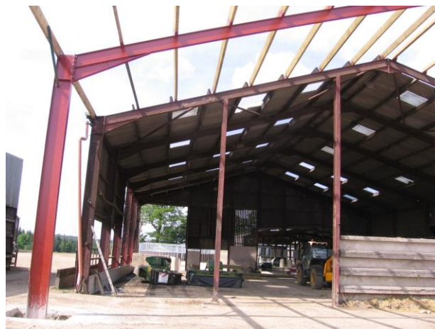
Photo shows the height of the roof from which Daniel Telford fell, narrowly escaping death.
