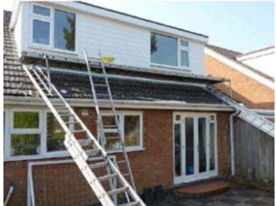
Inspectors intervened when they came across this unsafe construction site (above)
